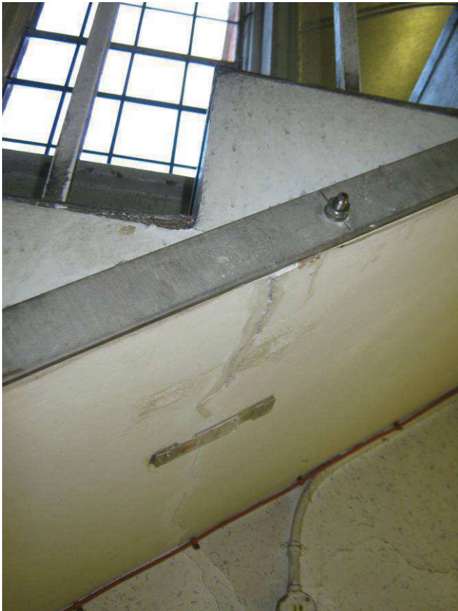
Photo 12. Cracking to soffit of staircase
